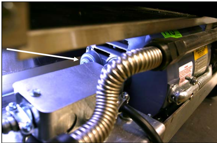
Filter Pump Reset Switch (Arrow)
